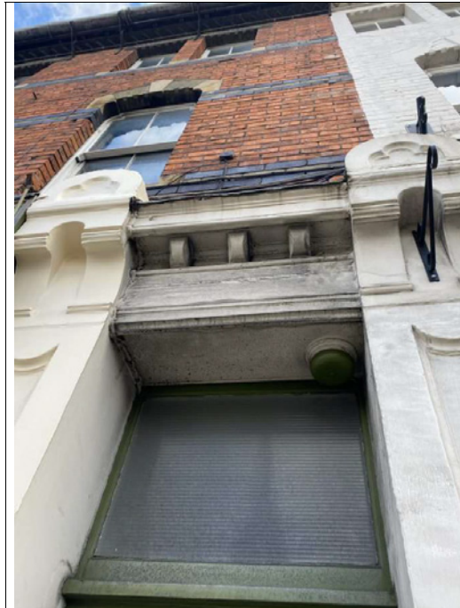
Overhead fascia, dentils and cornice to side door require redecoration.
