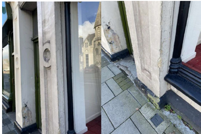
Pilasters in need of redecoration.
