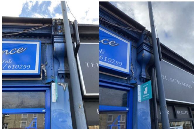
Right side corbel showing peeling paint, redundant metal bracket, obstruction of street lamp post and deteriorating timber of fascia.
