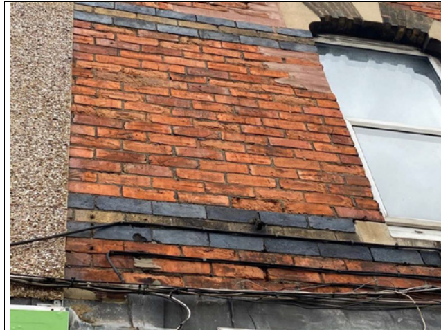
Deteriorating brickwork and congested building services.
