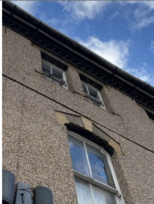
Poor condition of upper floor windows and failing rainwater goods along the roof edge.
