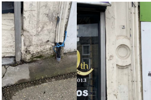
Left photo - Deteriorating lower pilaster (right side). Right photo - Cabling running over the pilaster surface and deteriorating surface condition (right side)
