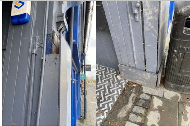
Left side pilaster obstructed by previous interventions – including boarding, tiling and boxed out with timber. Boxed out timber is deteriorating, particularly at the bottom. Street furniture (black plastic waste bin) is unsightly and obstructs features.
