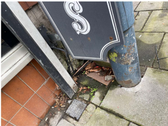
Deteriorated pilaster beside sign and behind lamp post.
