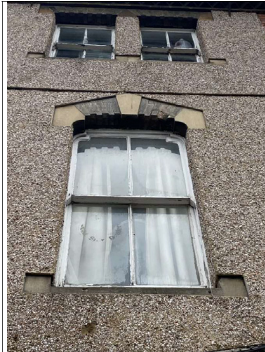
Poor condition of upper floor window. Ornamental lintel details in brick and stone remain visible.
