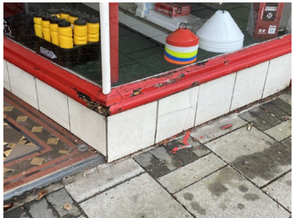
Timber decay to the stallriser nosing detail and a cracked tile.
