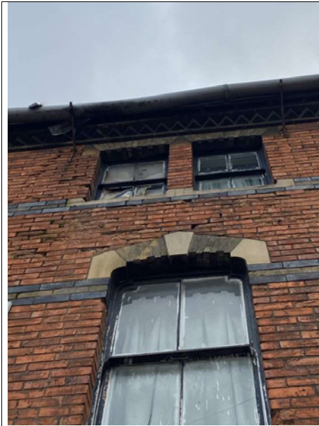
Poor condition of timber windows and broken guttering
