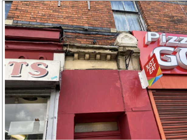
Original dentils and corbel over upper floor entrance door, possible indication that original features are behind timber box hoarding and shop fascia. Redundant hanging bracket. Note the weather covering over the awning is coming away and the timber above the dentils is deteriorating.
