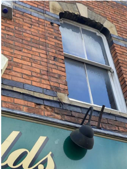
Brick Deterioration and trailing wire to upper façade.
