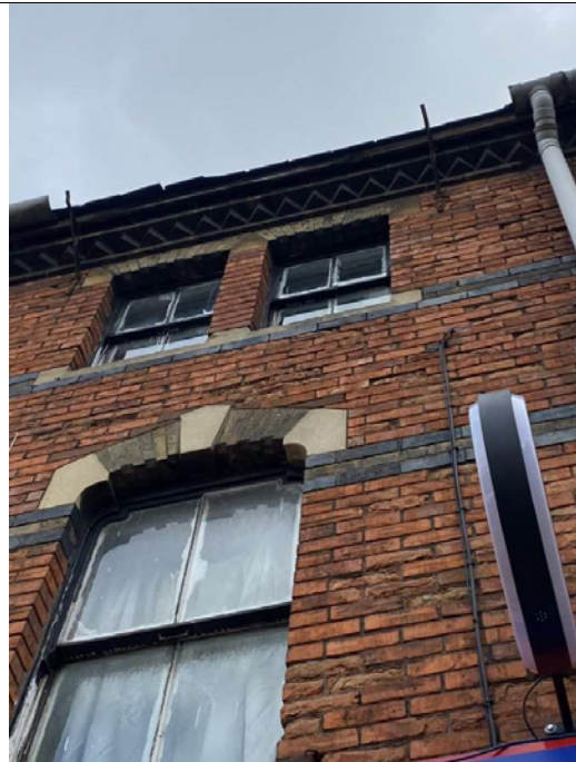
Missing guttering and insecure slates.
