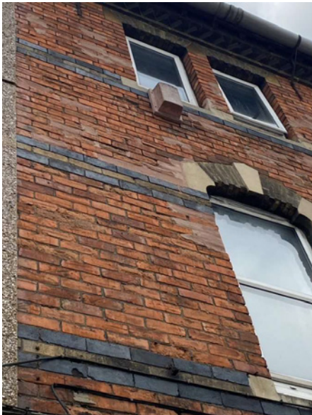
Platched repairs to deteriorated bricks, most likely cause is mortar repointing being too hard.
