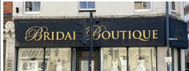
Oversized fascia sign obscures upper part of the original shopfront.
