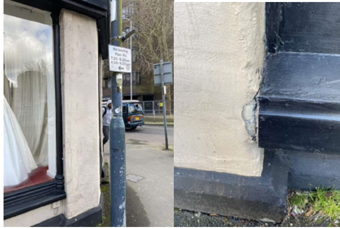
Shopfront pilasters with deteriorating paint.
