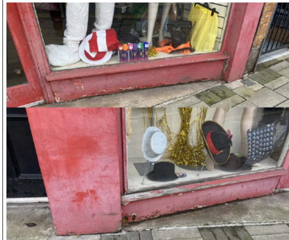
Deterioration to low stallrisers at the shopfront.
