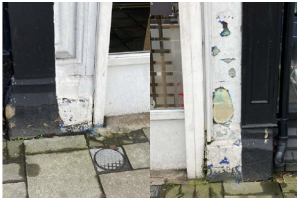
Left – deterioration of base of left-side pilaster.
