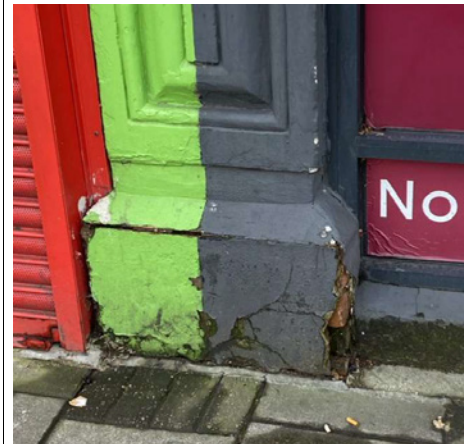
Base of left side pilaster deteriorated.
