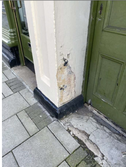
Failing paint at base of pilaster.
