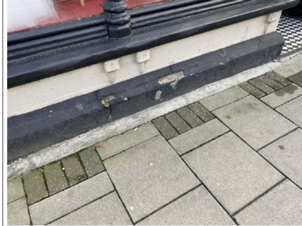
Damage to the nosing on the stallriser.
