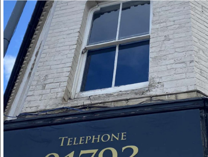
Timber windows to the upper floors, deteriorating paintwork and congestion of wires.
