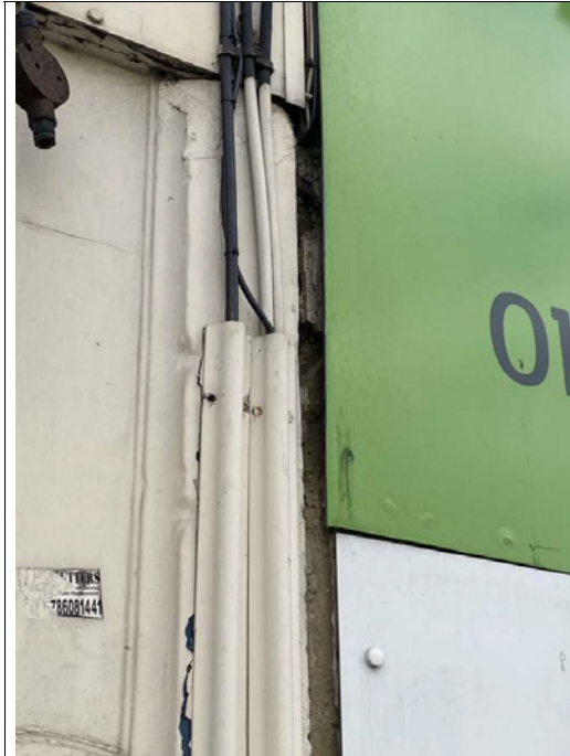
Conduits fixed to adjacent pilaster and some indication that the shopfront façade behind the modern signage is failing.
