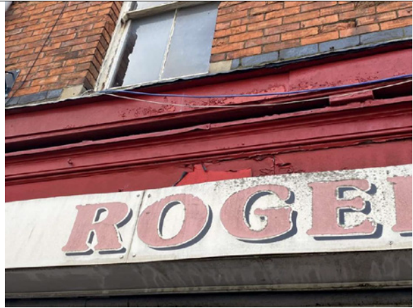
Peeling paint on the shop fascia and hanging wires.
