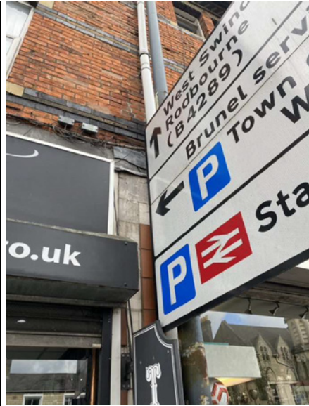
Missing tiles from right side of fascia. Corbel reinstatement would be ideal but this would require moving the highways sign.
