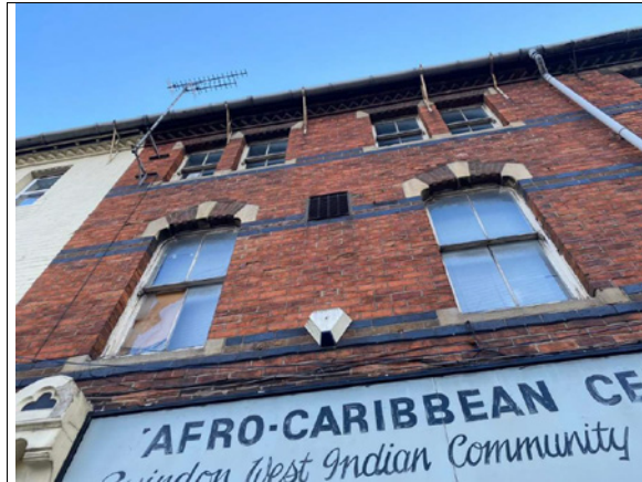
Upper facade showing poor condition of windows, trailing wires, alarm box and large vent between first-floor windows.
