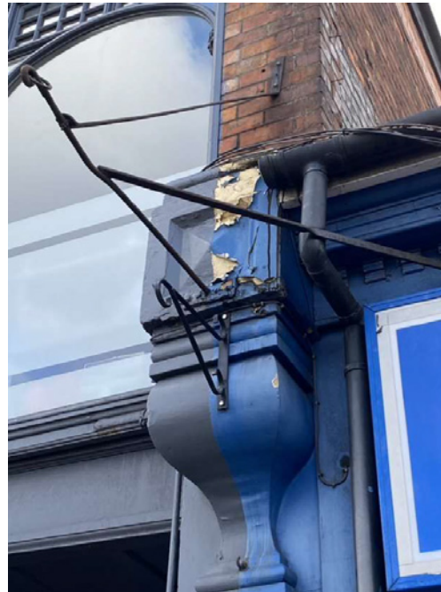
Left side corbel demonstrating peeling paint. The upper bracket is of some historic interest and is unique to the terrace. The lower bracket is a modern addition.
