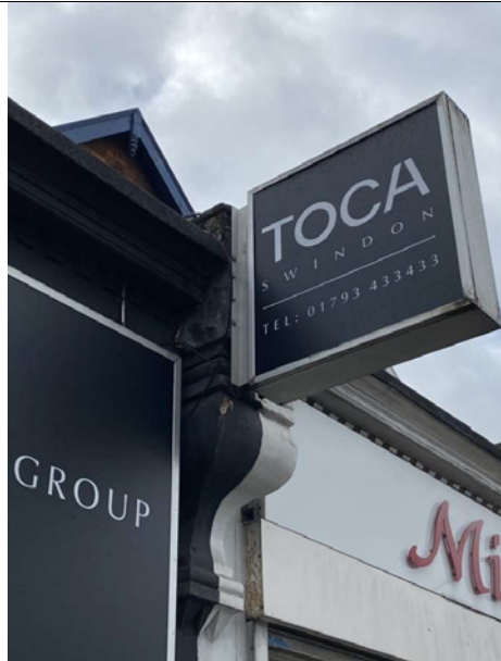
Photo showing intrusive fixing of shop sign over corbel and detail of covering over corbel top is inconsistent with exposed brickwork.
