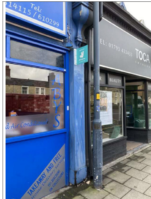
Timber boxing over original pilaster feature. Minor deterioration to bottom corners.
