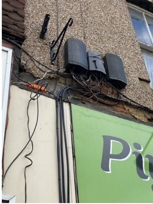
Congested building services and failed textured cement render allowing original brick façade to show through.
