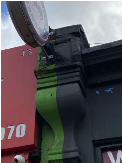
Deteriorated top of corbel over left side pilaster
