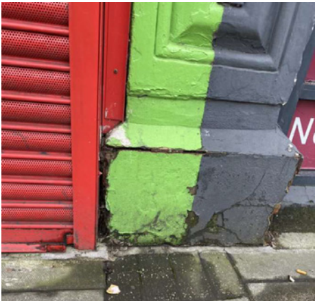
Photo showing deterioration of base of pilaster.
