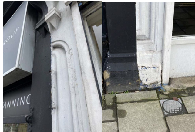
Photo showing delamination of the bottom of the pilaster and infill of the pilaster moulding.
