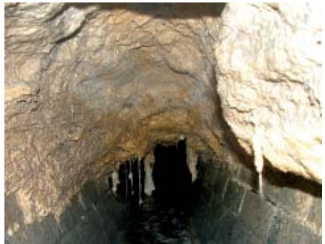
Fat beginning to block a sewer
