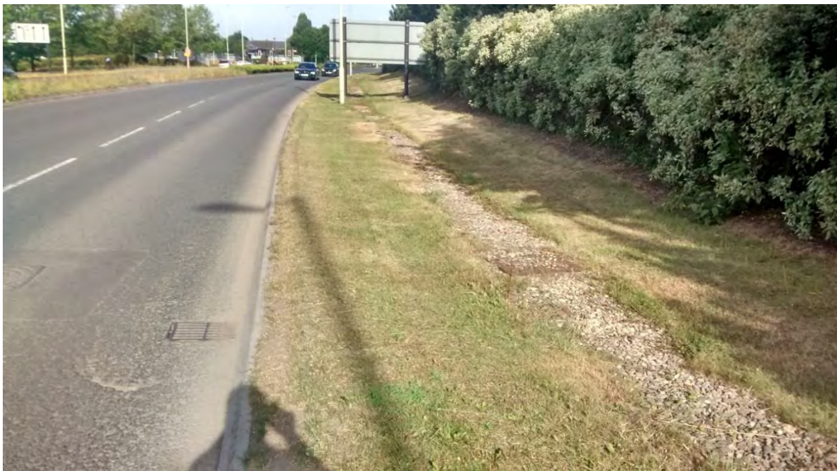
Figure 29 Filter drain not providing drainage for highway
